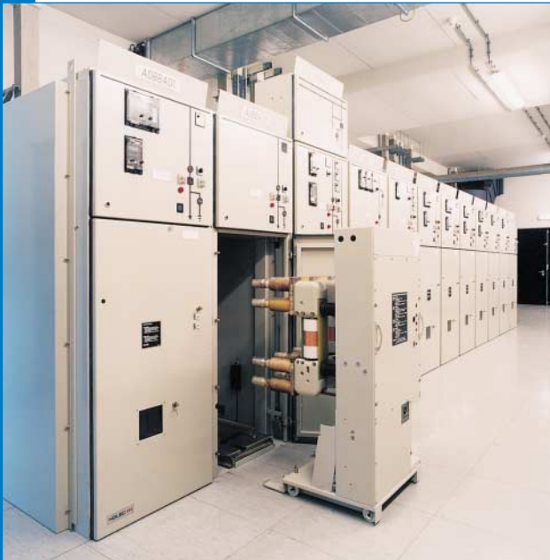
Unitole Type UP distribution system.
