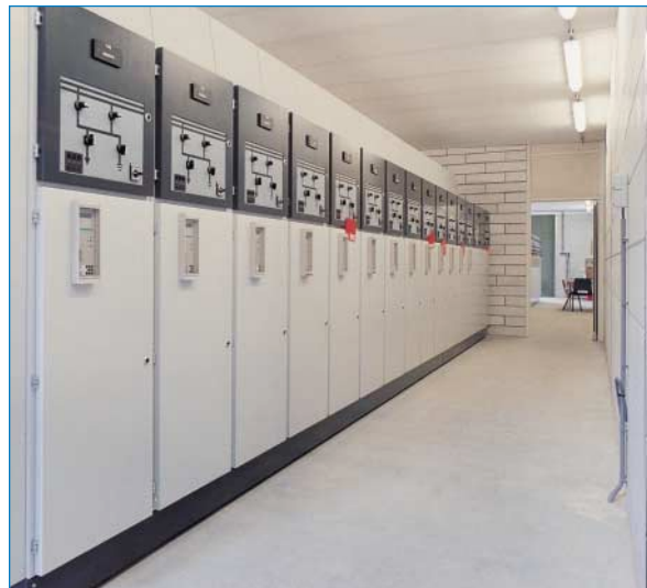
Turnkey project at Essent in Emmen, The Netherlands.
