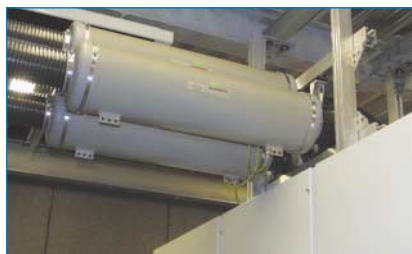
Duresca busbar connection.
