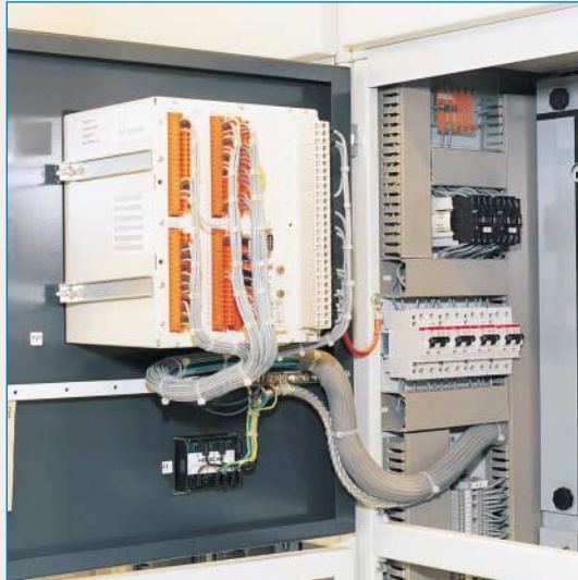
Inside of panel door with secondary and protection relay.
