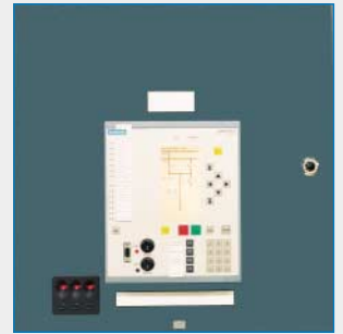
Siemens type Siprotec protection relay.
