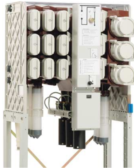
Magnefix type MD4 circuit-breaker protected tee-off.
