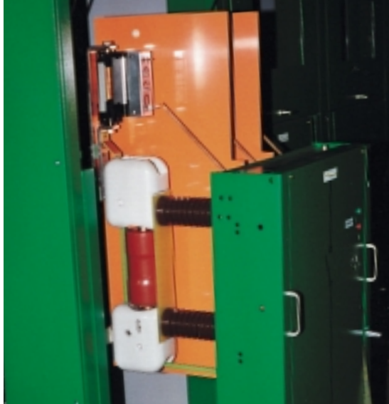
Holec vcb with primary protection relay in 24 kV switchboard of Huser, Switzerland
