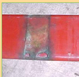
Tracking on a busbar duct
