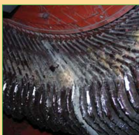
Corona damage to motor windings
